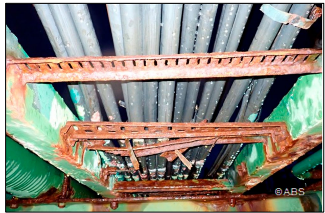
Corroded cable tray support on deck
