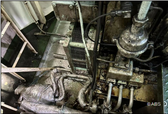
Generator engine fuel pipes leaking
