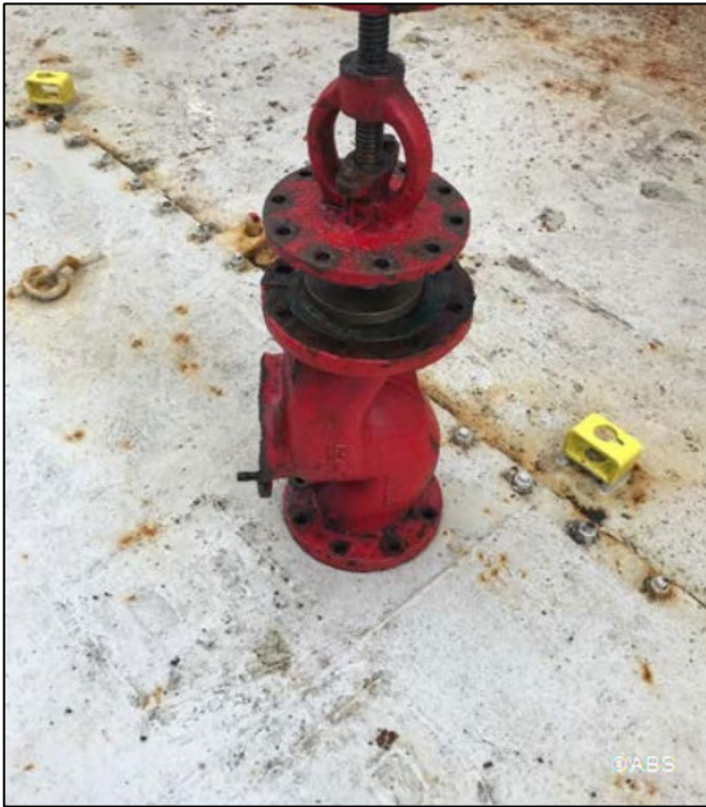
Engine room fire main isolating valve –malfunctioned
