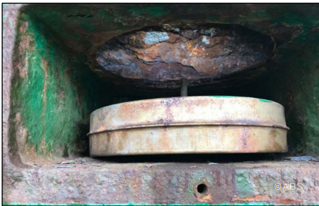
Ballast water tank vent head wasted and seal missing
