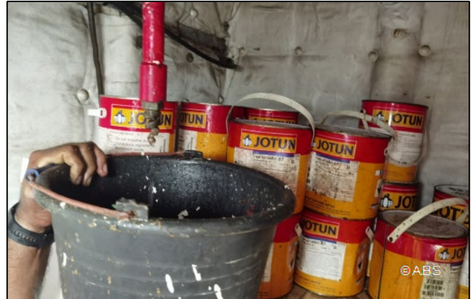
Paint store sprinkler head found clogged
