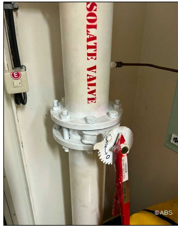
Main fire line isolation valve non-functional
