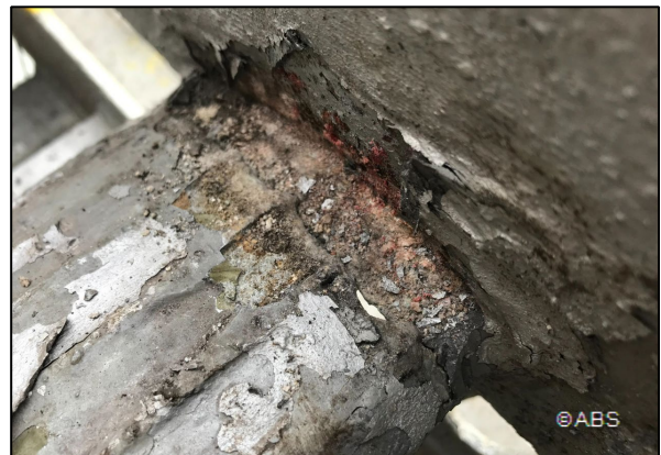
Crack accommodation ladder with waste
