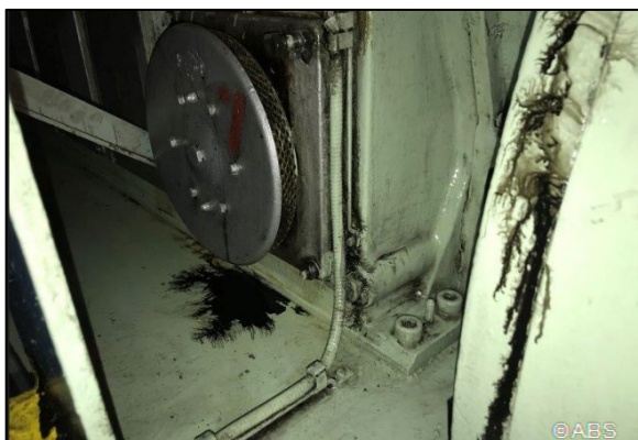
Oil leakage from generator engine crank case explosion door and fly wheel end seal
