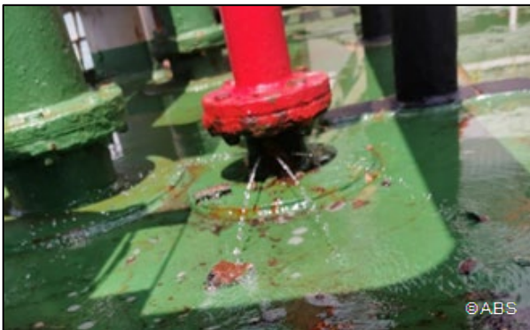
Fire line on main deck excessively corroded with hole
