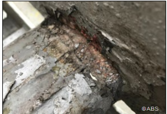
Wasted and fracture section of accommodation ladder
