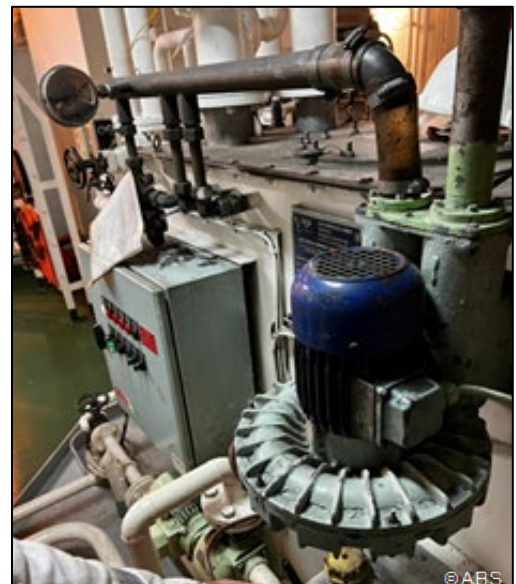
Sewage treatment plant not operable
