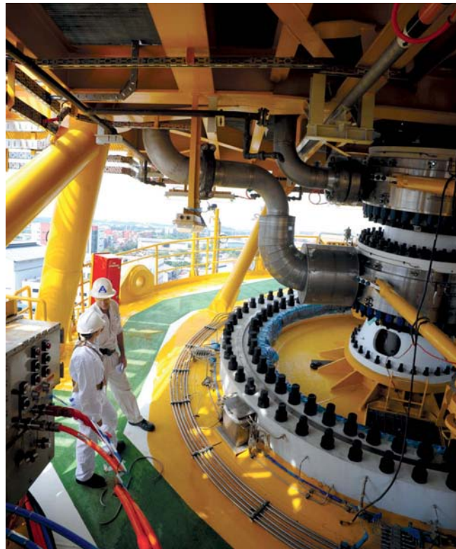
Mooring systems are among the critical components that must be evaluated carefully when considering FPSO life extension (photo: Andre Eichman)
