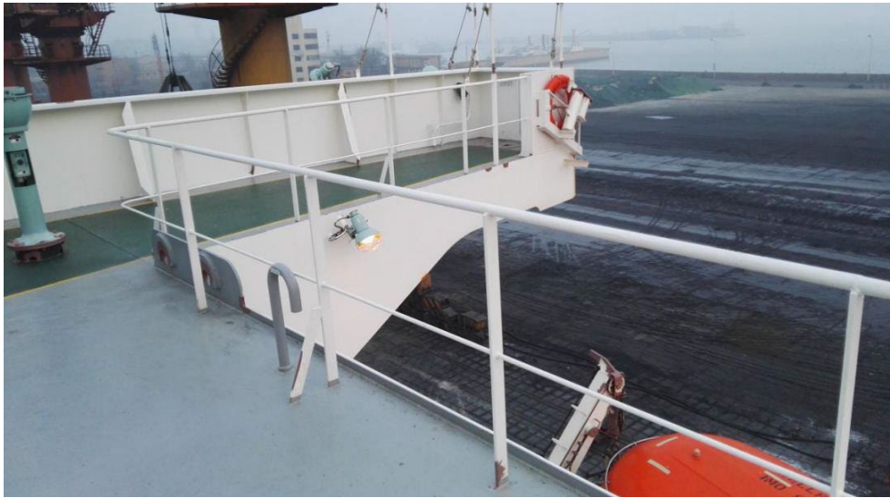
Figure 2 Guardrails with two courses on the open part of deck structure ( SDC 10/11).
