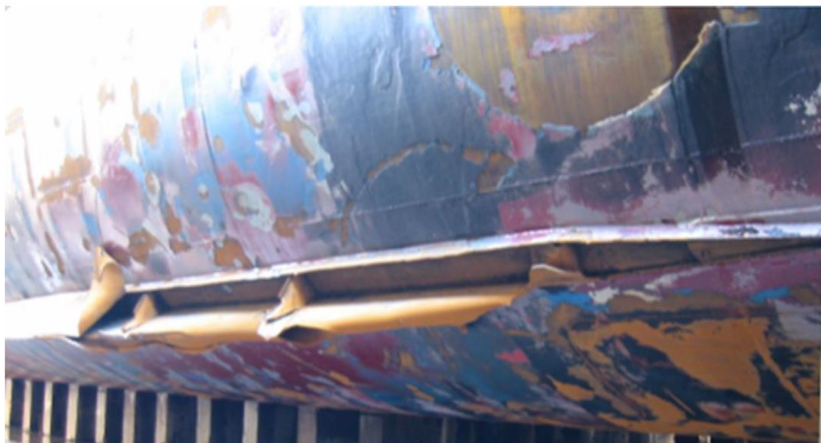
FIGURE 15 Damaged Bilge Keel
