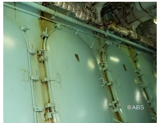
Sign of fuel oil leakage over main engine crankcase door
