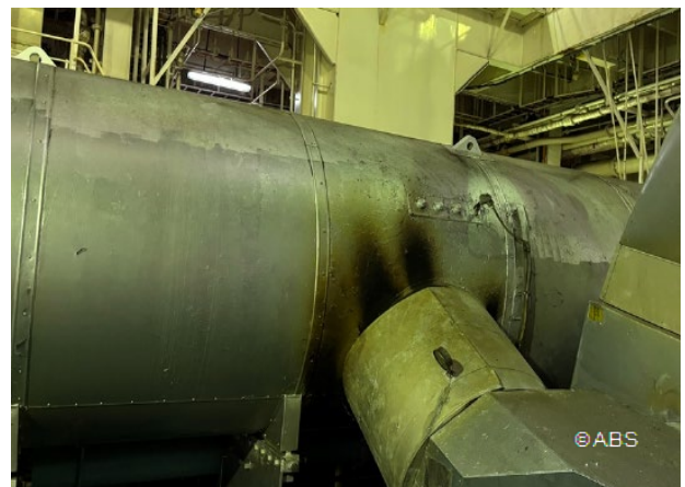
Sign of exhaust gas leak at main engine exhaust gas trunk
