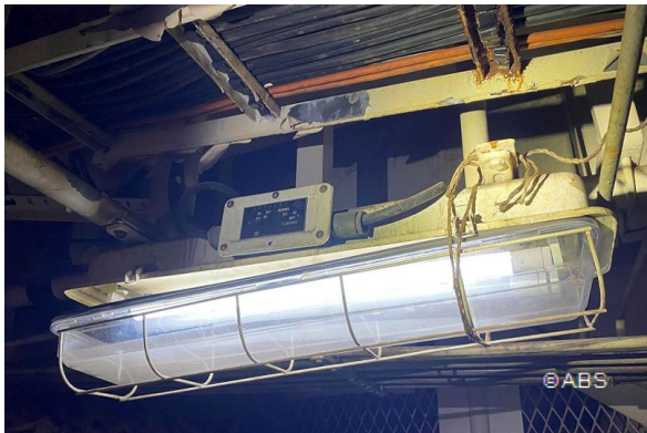
Electrical fixtures are not secured properly
