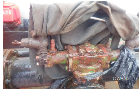
Hydraulic actuating mechanism for bunker line valve wheel wasted and broke while operating
