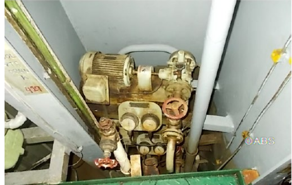
Stern tube tank gauge glass unable to read
