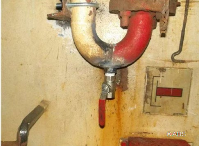
No drainage arrangement is provided at the bottom of the U-shape fire line on both sides of the main deck. Picture posted after rectification of finding.
