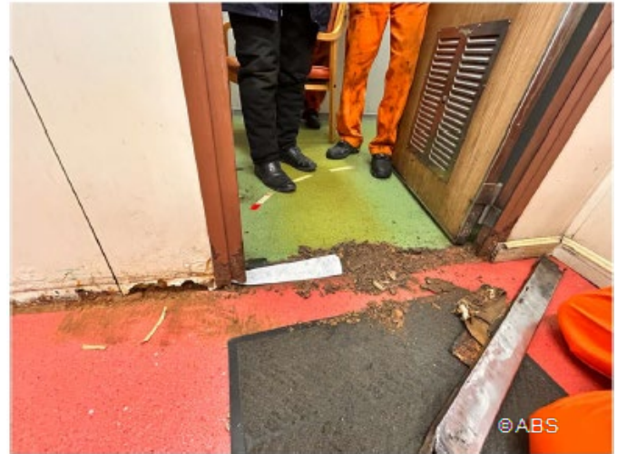
Crew mess room entrance door sill (Class-B fire door) and bulkhead panel wasted. Fire boundary integrity lost.
