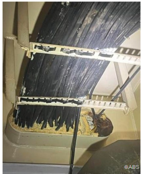
Multi-cable transit in the Engine Room workshop not as required – cable is run outside of the cable transit and improperly sealed.
