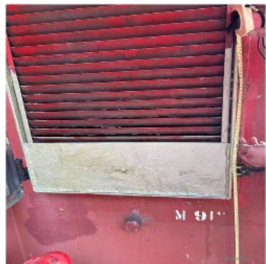
Height of the ventilators at poop deck was modified to 900mm. The original height during PSC inspection was 720mm. Per Load Line Convention/Regulation 19, ventilators in position 1 shall have a coaming height of at least 900mm.
