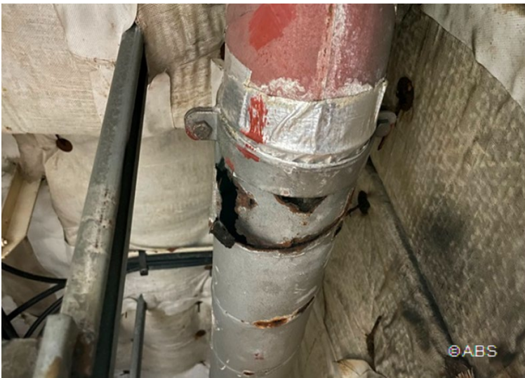
Holed ventilation ducting.
