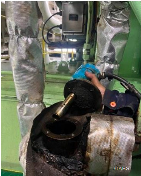
Top cover of Main Engine Fuel Oil leak-off alarm bypassed. Sensor was removed from alarm assembly.
