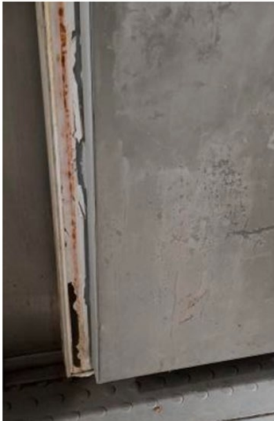
Refrigerator – meat room door gasket rubber is deteriorated.
