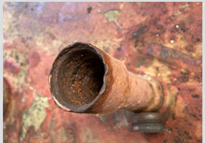
Sounding pipe closing cap thread damaged
