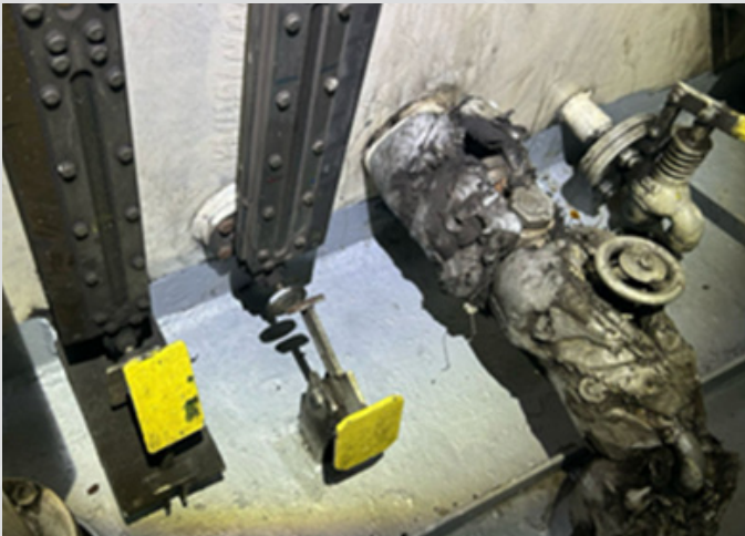
Quick closing valves for lubricating oil system and marine gas oil system blocked permanently in open position. Steam line insulation is not maintained.
