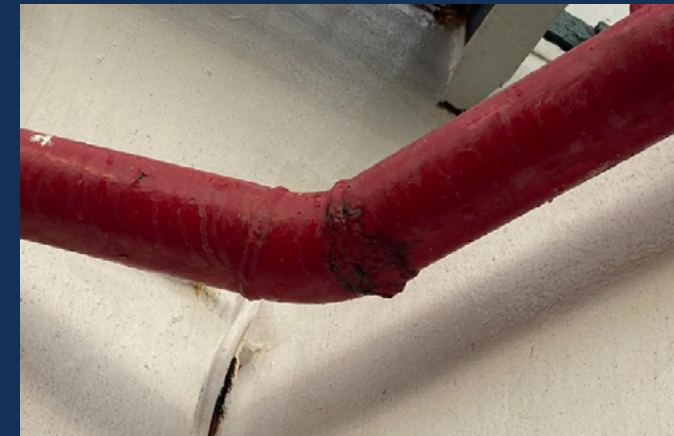
Figure 1: Corroded fire pipe on navigation bridge.
