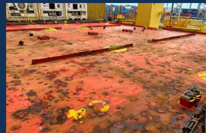
Figure 4: Hatch cover gaskets were found defective.
