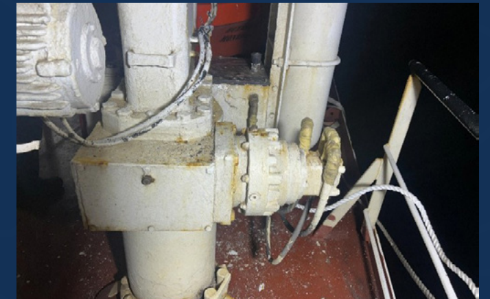
Figure 2: Temporary repair on corroded hydraulic oil pipe joint for rescue boat launching arrangement.
